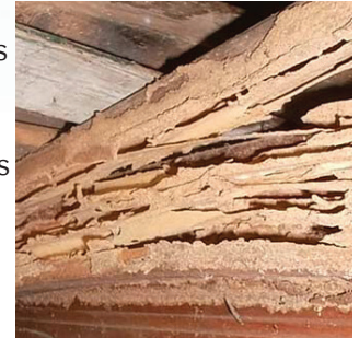
Subterranean floor joist damage
