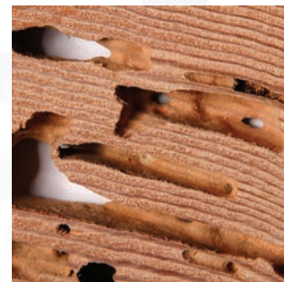
Drywood termites can eat the inside of a beam, leaving the entire exterior untouched.
