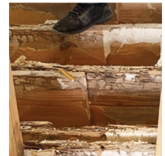
Joist damage under spray foam
