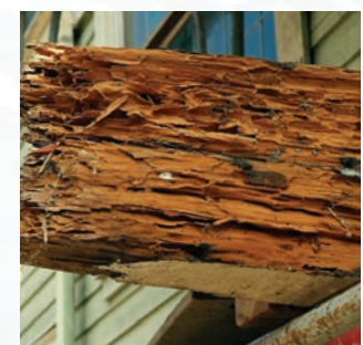
Formosan termite damage
