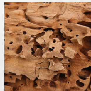
Carpenter ants excavated gallery in wood
